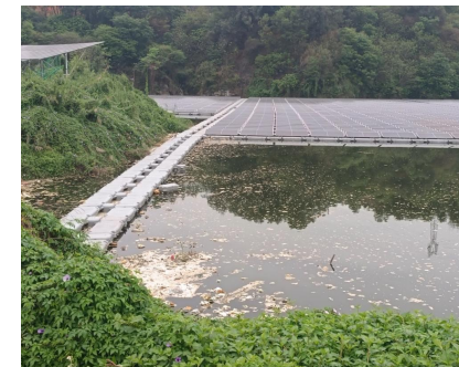
Big lake-Cable landing and maintenance walkways
