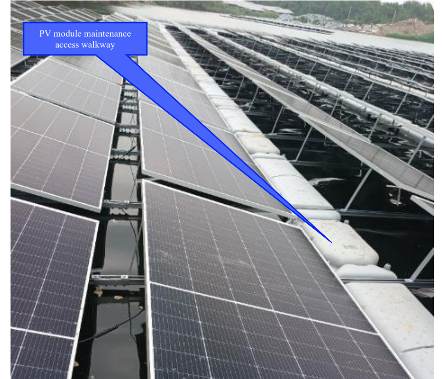
East-west maintenance access walkway
